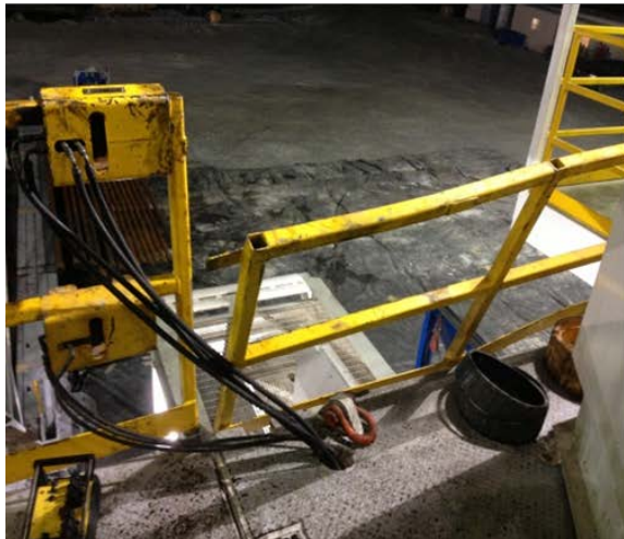
Damage to Handrail
