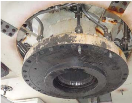
Upper half of failed LMRP Connector
