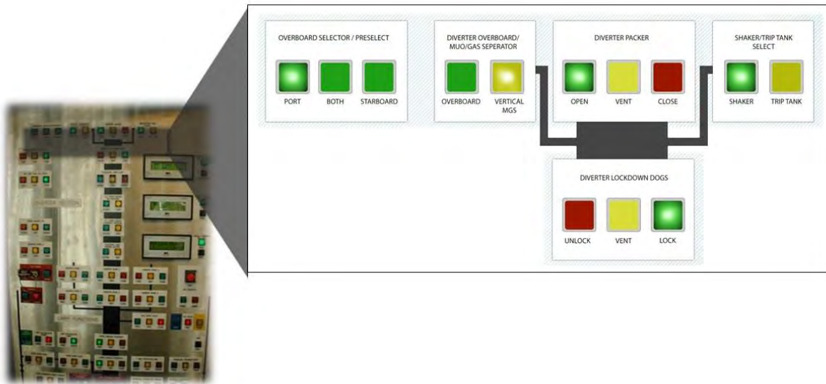
Figure 1-1. Control panel (left) and partial close-up of control panel on the Deepwater Horizon found in the driller's cabin 48 and on the bridge of the rig. These controls were used to preset the diverter.
