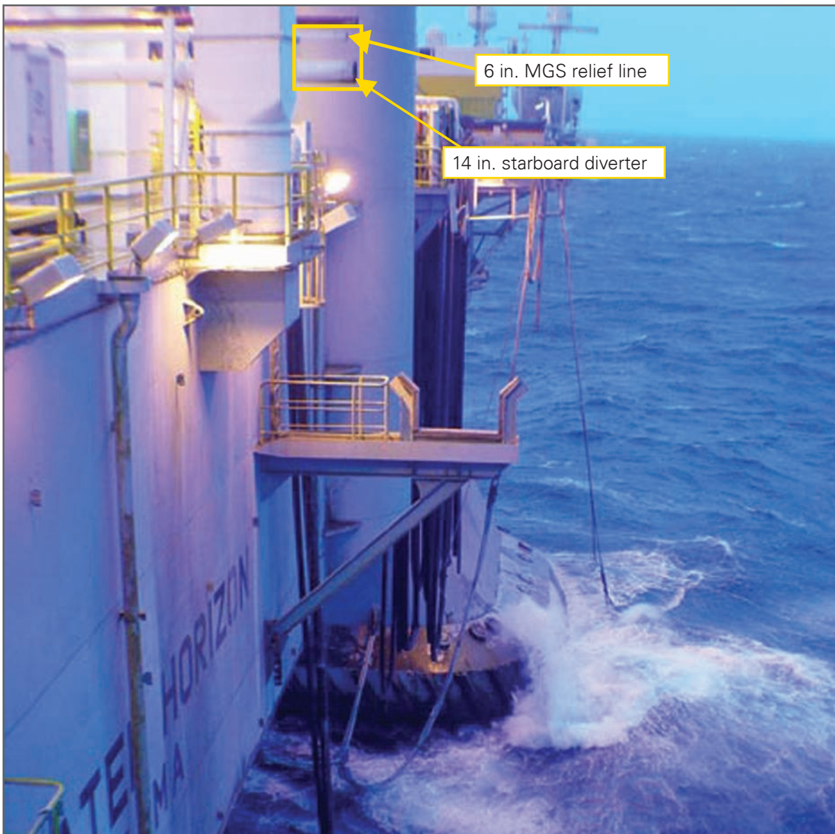
Figure 6. Photograph of Starboard Overboard Lines.
