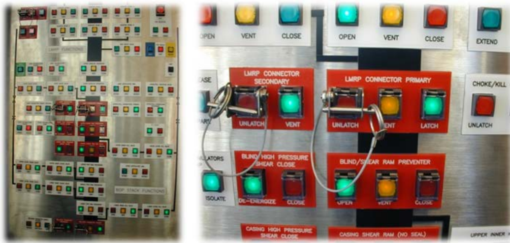
Figure 2-4. Control panel (left) and partial closeup of control panel on the Deepwater Horizon found in the driller's cabin and on the bridge of the rig. These controls are used to activate the BOP. 12
