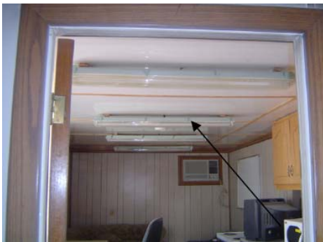
Normally used light fittings
