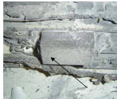
Overheated ballast (main cause of fire)
