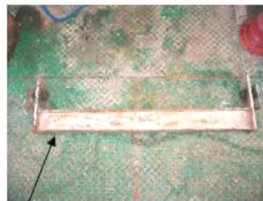
Stopper plate not in position
