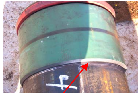
Note the beveled collar shoulder.
