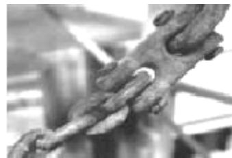
Another Unacceptable Twin Clevis Link
