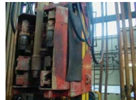
Picture showing rubber mats attached to PHM carriage, to assist in containing hydraulic leaks within carriage assembly.
