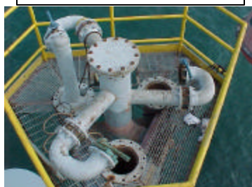
# 1 Deep Well Tower Crows Nest
