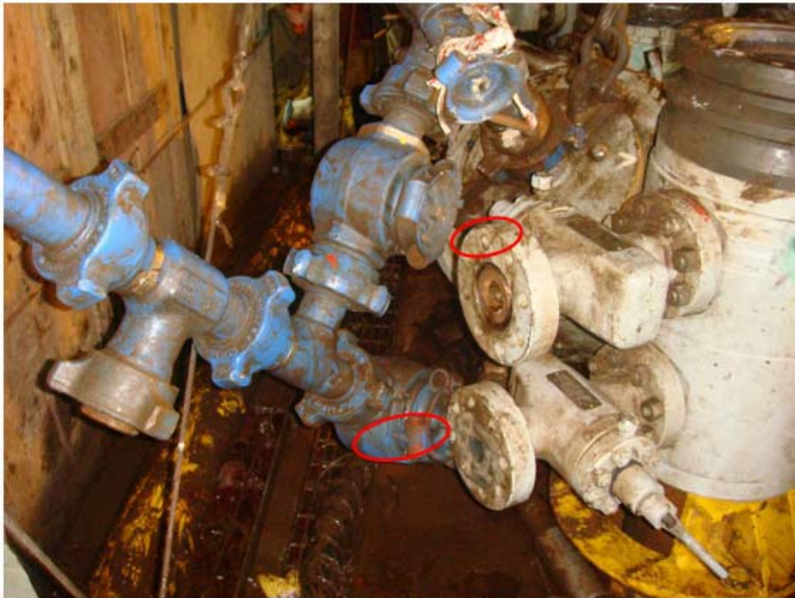
Photo 1 – approximate Crush points between annulus valve and valve (1) on cement head
