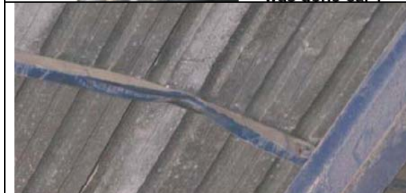
Cross-beam of the roof struck and dented from impact of the wheel (Tyre-Rim Assembly) launched from the floor (ca. 8 mtrs)
