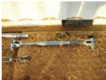
Improper rigging screw
