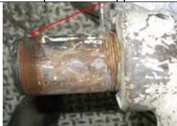
Only three threads were buried into the receptacle on the standpipe.
