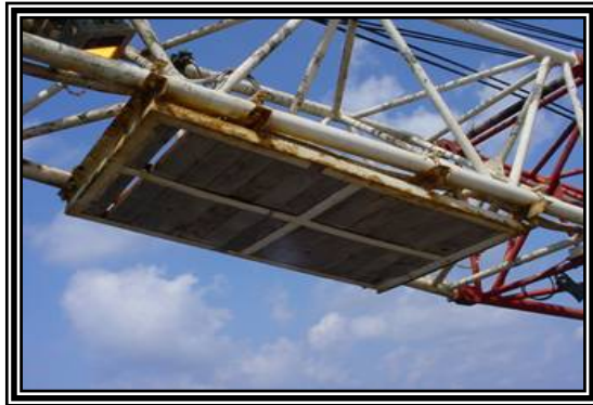
Fig. 4: The boom saver pad that did not prevent main block from contacting the boom.
