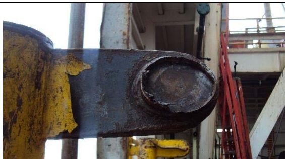
Port V-door King Post after the pipe broke.
