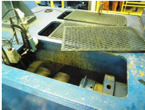
Pony Rod Cover Loose on top of the mud pump.
