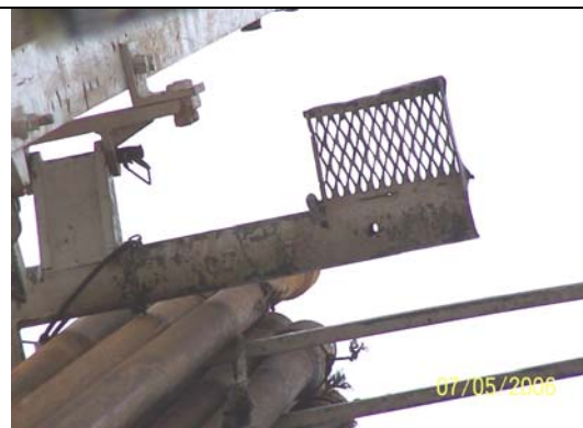
Photo 2 – Area of derrickboard from where Slide Bar fell
