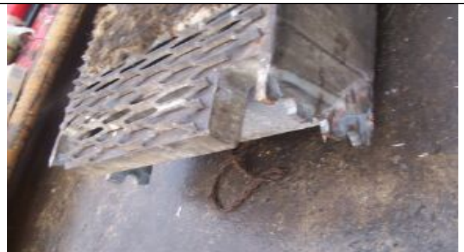
View of broken diving board padeyes
