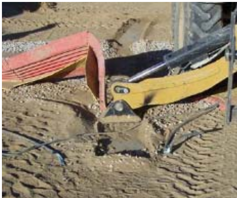
Cut Electric Cable
