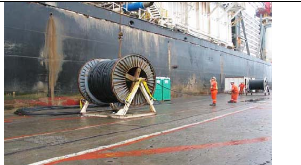
Use of rig crane and soft-line arrangement with Personnel kept at a safe distance.
